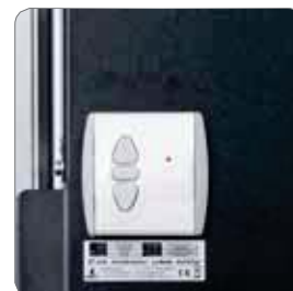
Electric control panel
